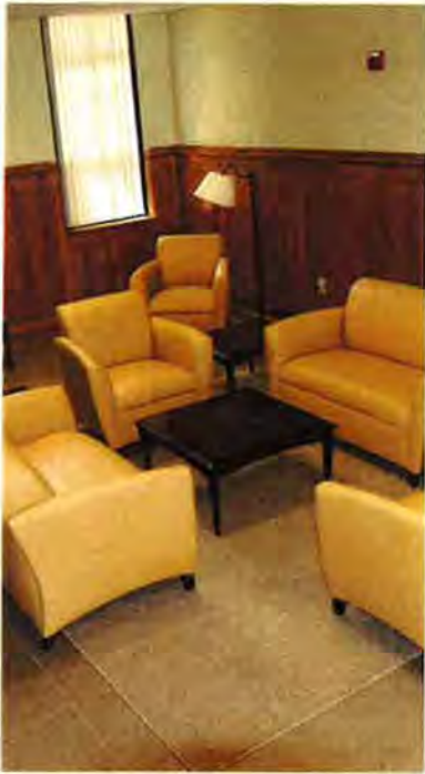
Summer 2010 renovations in the first floor Tolbert lounge and common area restored original, historic wood paneling.
